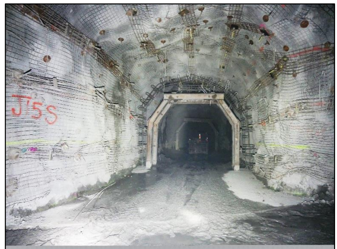
Figure 3. An example of ground support in the B3 extraction level, short and long support are installed including pillar wrapping. A drawpoint steelset is standing ready to be sprayed in with shotcrete.
