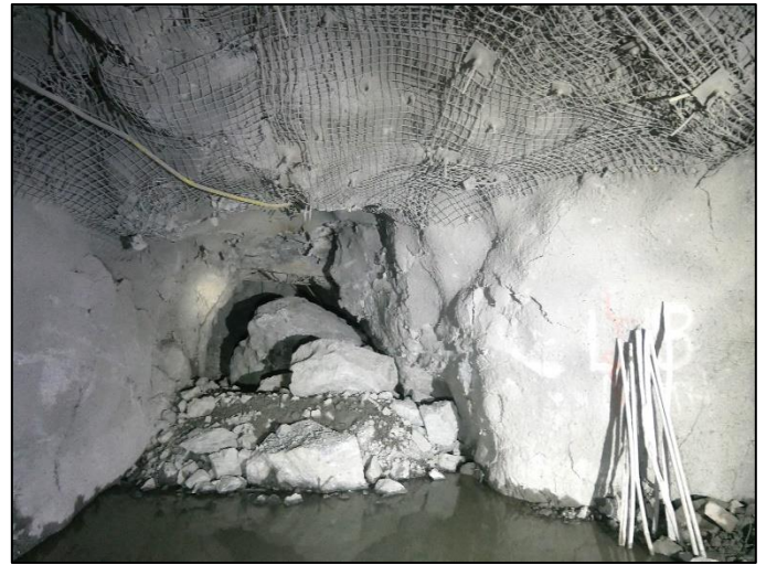
Figure 12. L18-N drawpoint in October 2023 prior to being closed. Ground movement and resultant damage can be seen in both walls and the back, with the right wall encroaching on the drawpoint opening.
